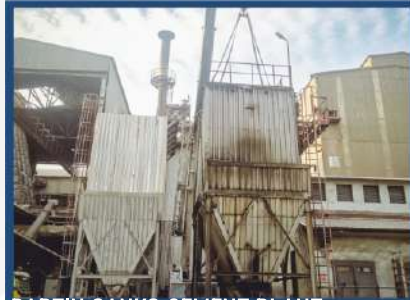
BARTIN SANKO CEMENT PLANT The old dust collection system was dismantled, and a new dust collection system was manufactured and installed.
