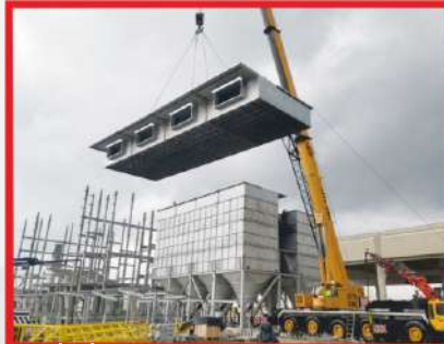
DENİZLİ ACARSOY ENERGY Manufacturing and installation of the dust collection system were carried out.
