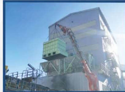
ENERJİSA TUFANBEYLİ Two dust collection systems were completed on a turnkey basis.
