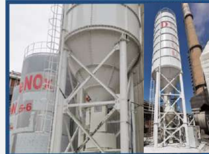
SOMA TERMİK SNCR – SCR (DeNO x ) systems were installed.
