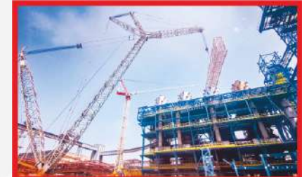
EKON – İSDEMİR 1. YF Together with EKON, we completed the fabrication and installation of the pipe rack piping for İSDEMİR Blast Furnace 1 YF.
